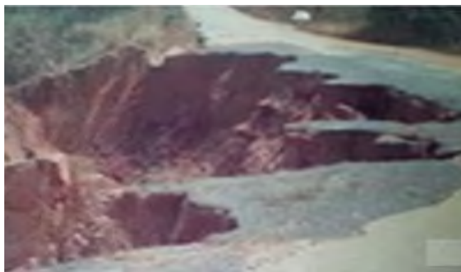
Photo xxii: Gully erosion causing road failure
